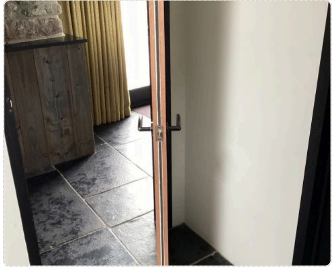
Ground-floor doorway · Intumescent strips / seals
