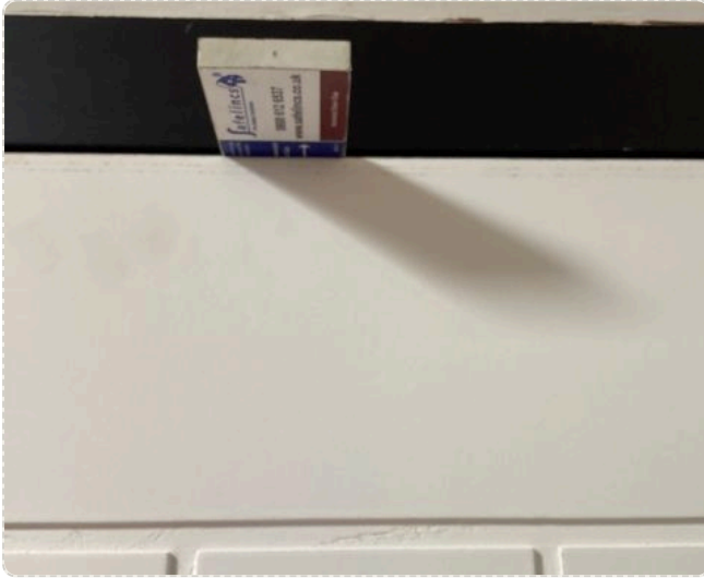
Ground-floor doorway · Gaps
